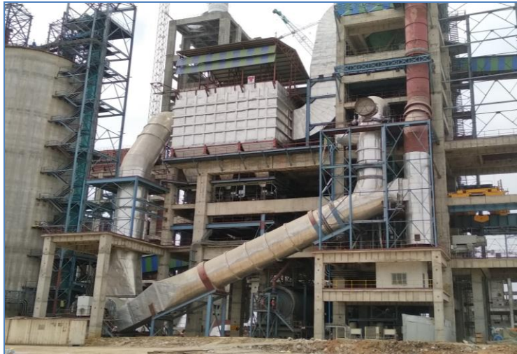
Cement Mill Main Bag house
