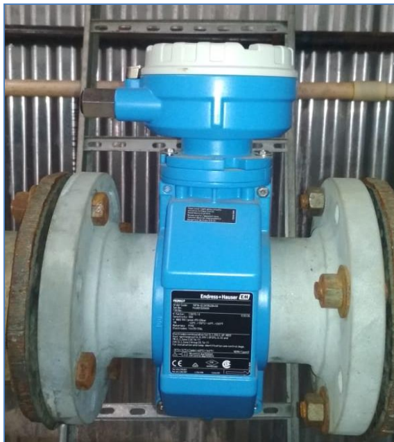
Flow meter for domestic consumption
